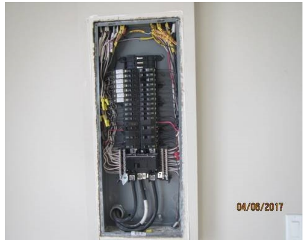
Open Electrical Panel
