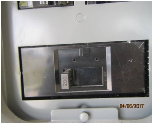
Main Electrical Disconnect
