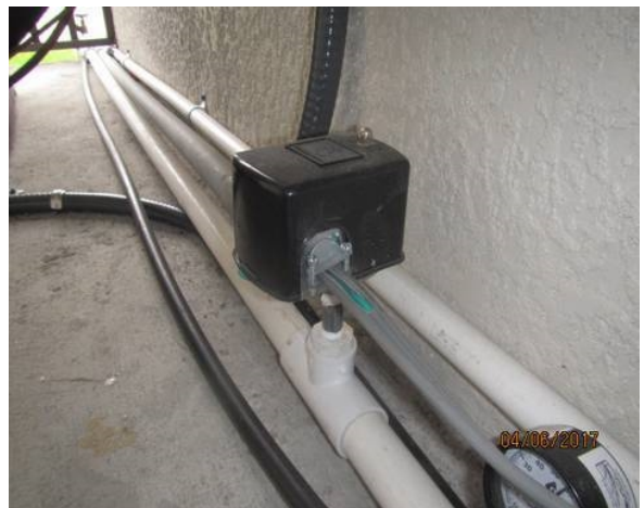
Cord Protector Not Secured Properly @ Well Pressure Switch
